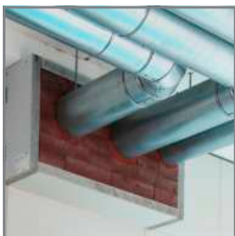
■ Pipe and cable bulkheads
