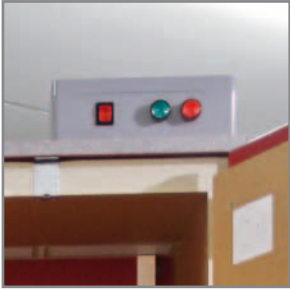
Control unit with fire detection
