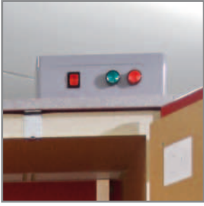
Control unit with fire detection Malfunction message via optical signal and switch-off of the ventilation system.
