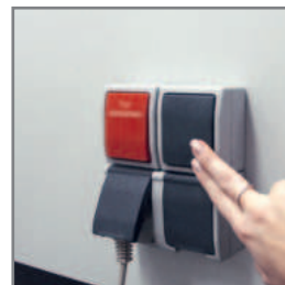
■ Switches, wall outlets
