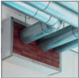
■ Pipe and cable bulkheads
