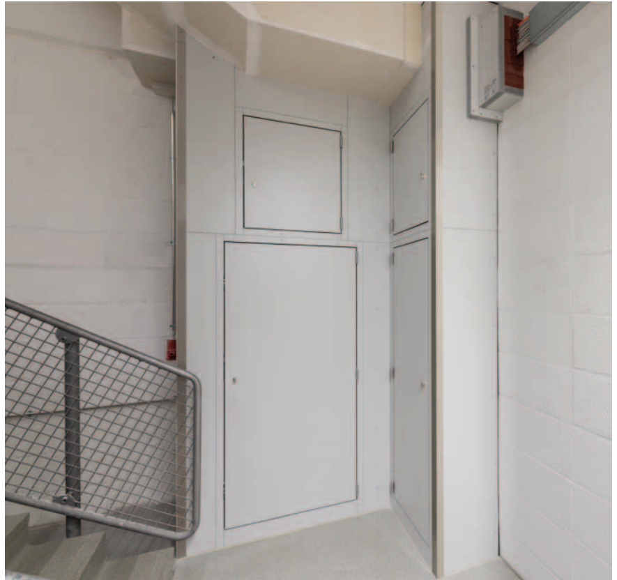
The fire hazard of the electrical distributors was safely separated from the stairwells in terms of fire protection.
