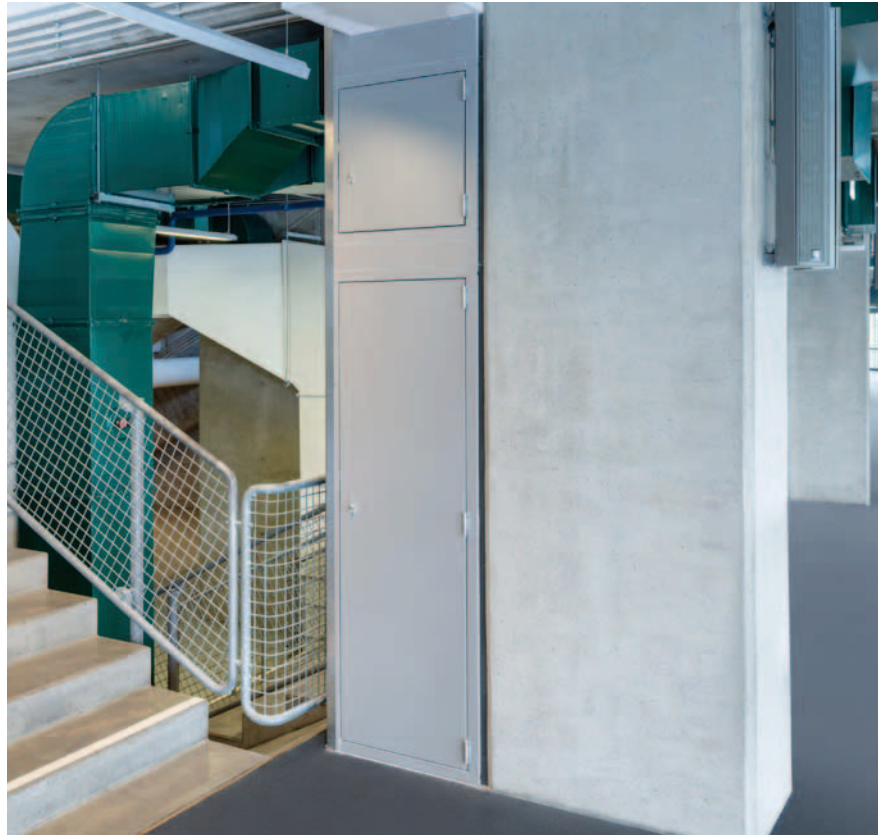
Room-high distribution boards in the escape route area, fire-resistant partitioning
