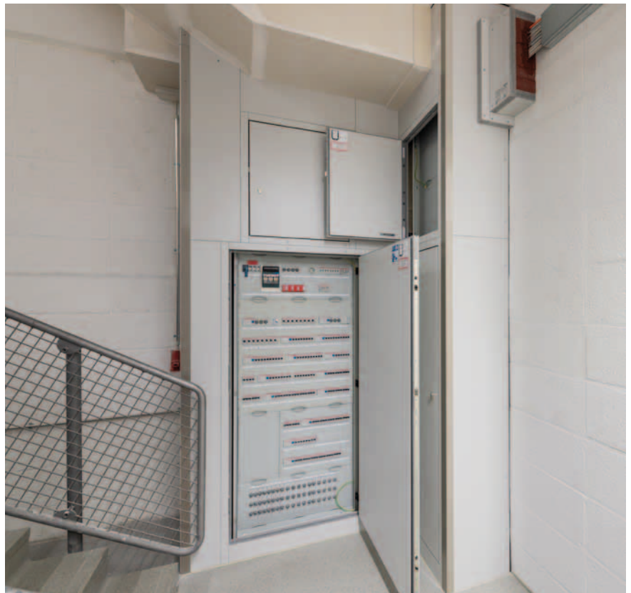
The fire hazard of the electrical distributors was safely separated from the stairwells in terms of fire protection.
