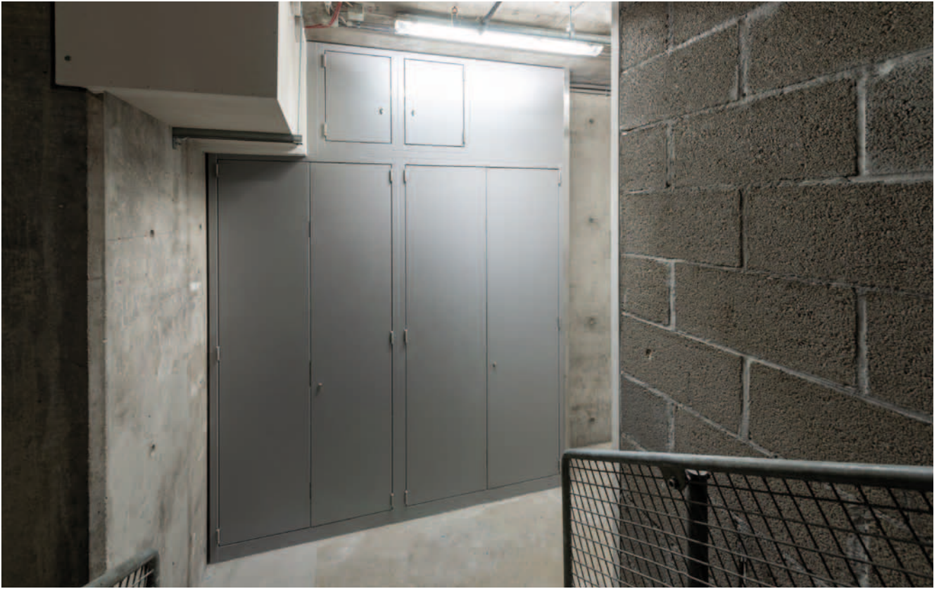
The fire hazard of the electrical distributors was safely separated from the stairwells in terms of fire protection.
