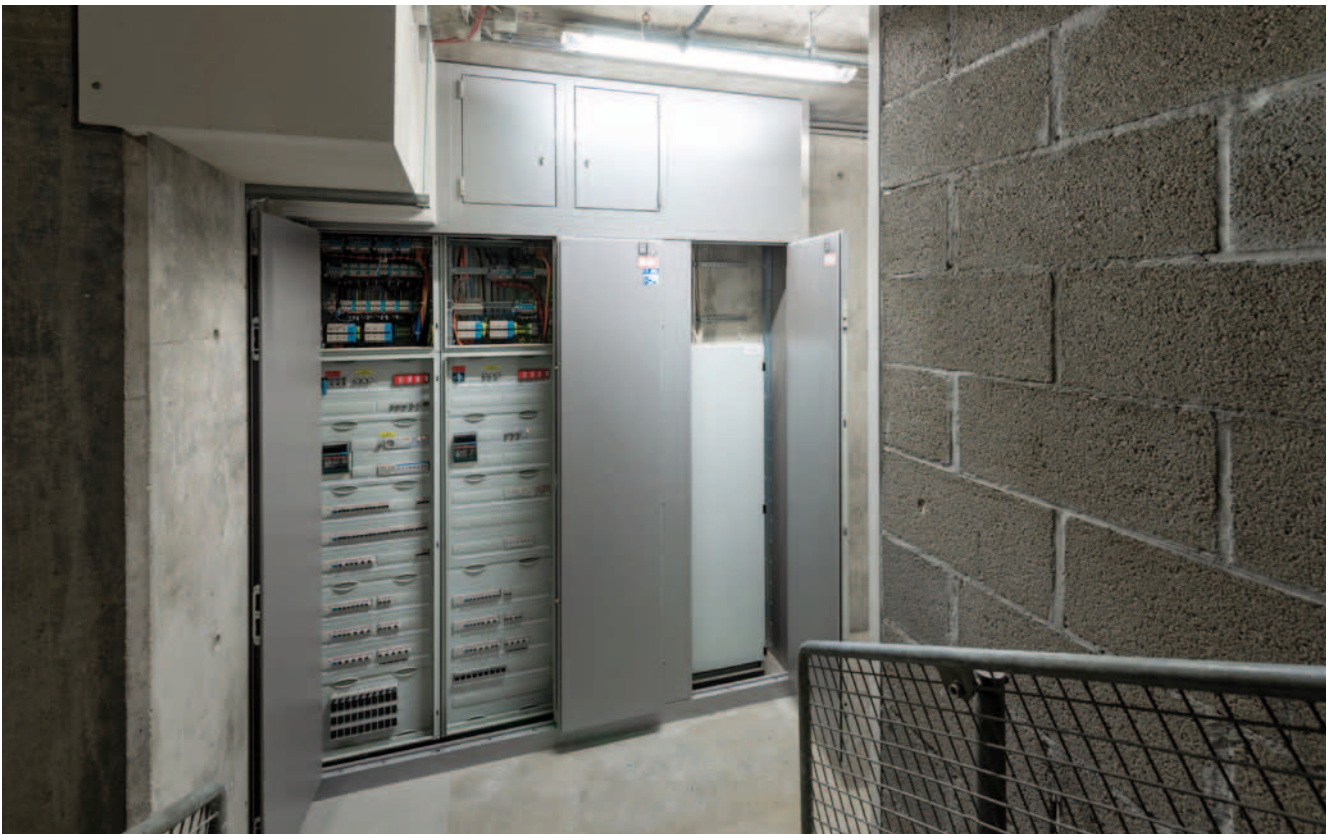
The fire hazard of the electrical distributors was safely separated from the stairwells in terms of fire protection.
